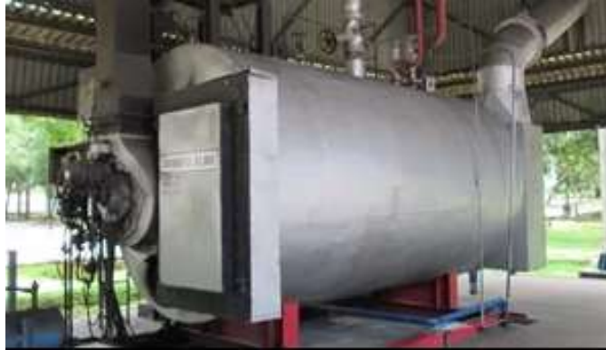
Figure 1. Boiler for a waste treatment system with improved temperature control.
